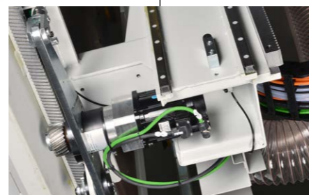
Lower gantry motor
